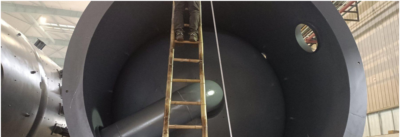
Inside a column: internals check
